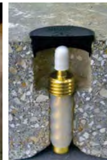
Sub-Slab Soil Vapor Pin
